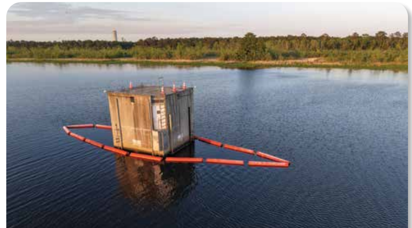
The CWS intake at Bushy Park Reservoir collects raw water and sends it to the Hanahan Water Treatment Plant.
