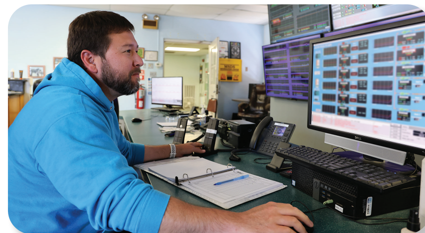
Operator Apprentice Kenny Soos and the other operators monitor numerous aspects of water treatment from our process control room.
