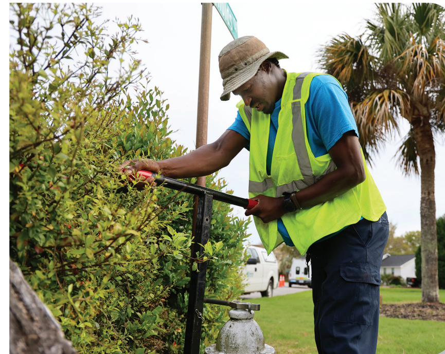
Hydrant Maintenance Operator John Bennett and his crew team members have to open fire hydrants to flush them.
